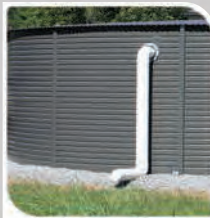
6-Inch Overflow Drainage Pipe
