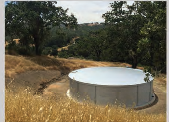
Fire Protection Tank for the Lago Giuseppe Winery
