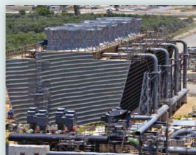
Cooling Tower Water Treatment
