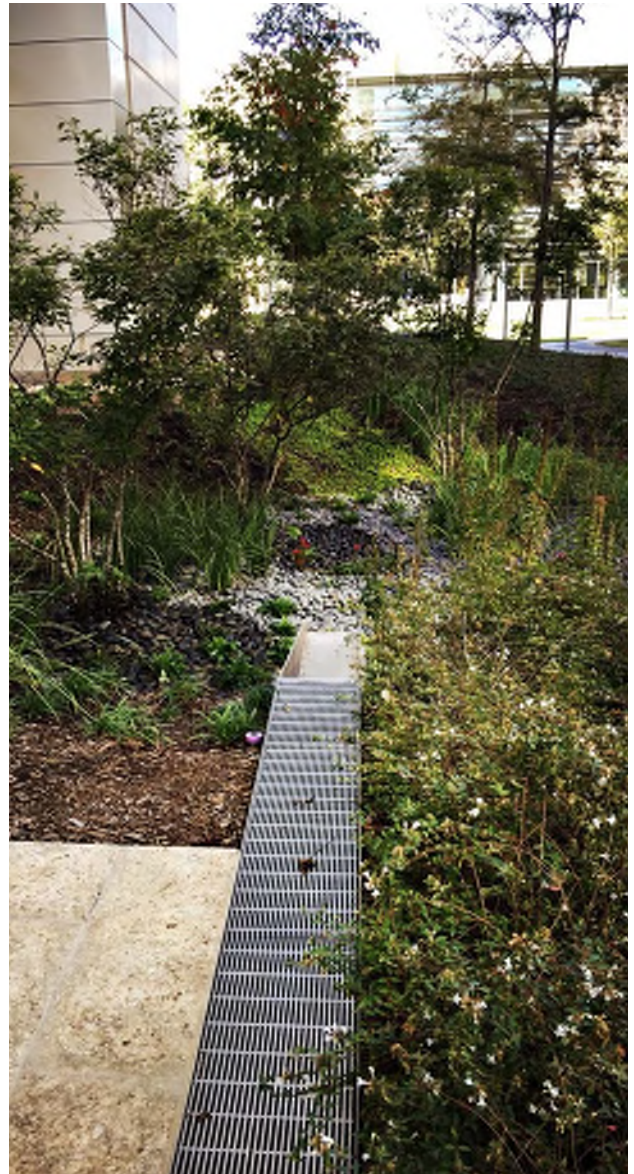
ABT's stainless tunnel installed in a rain garden
