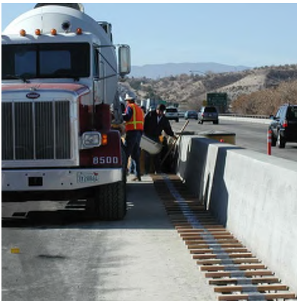
Highway barrier drainage
