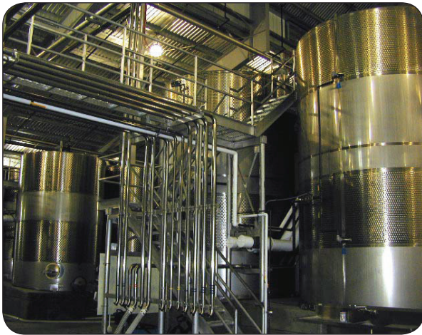
Connector Station and Fermentation Tanks
