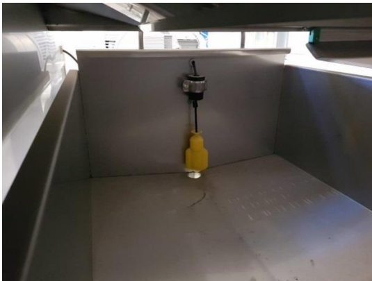
Must hopper level control
