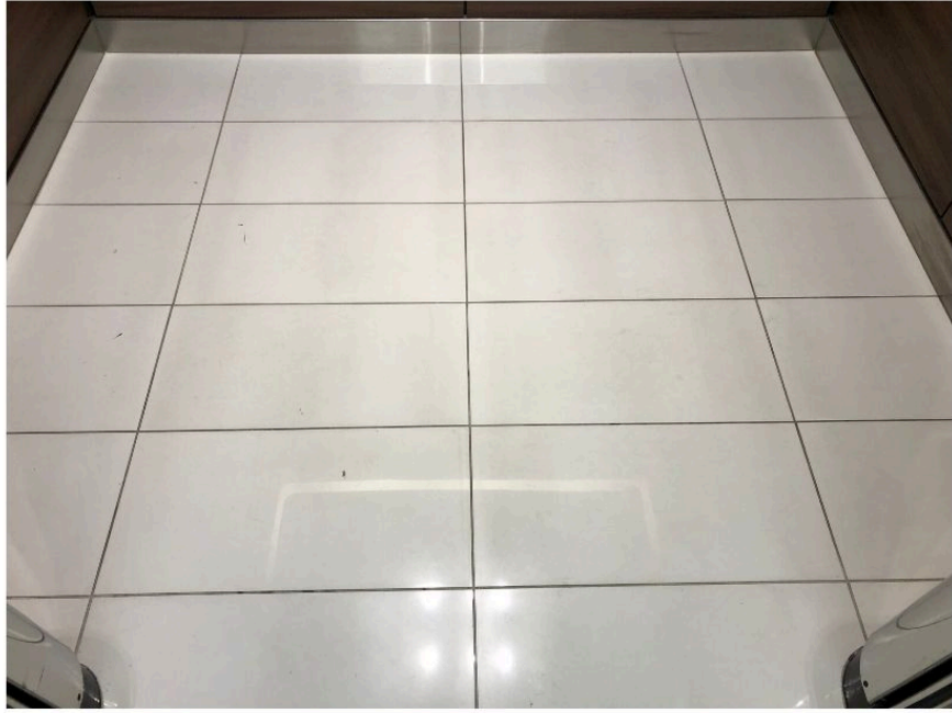
Before Cleaning & Grout Recoloring
